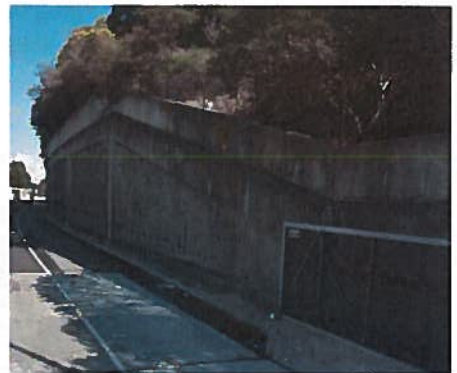
Eastbound I-580 requires widening in Contra Costa County to accommodate the third eastbound lane. The retaining wall shown must be removed and replaced with a wall set further back from I-580.
