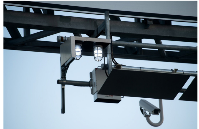
Close-up of toll system equipment under sign (enforcement beacons, reader antennae and laser trigger)
