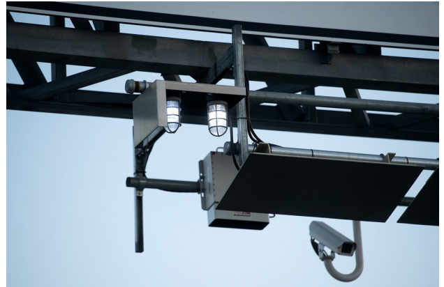
Close-up of toll system equipment under sign (enforcement beacons, reader antennae and laser trigger)
