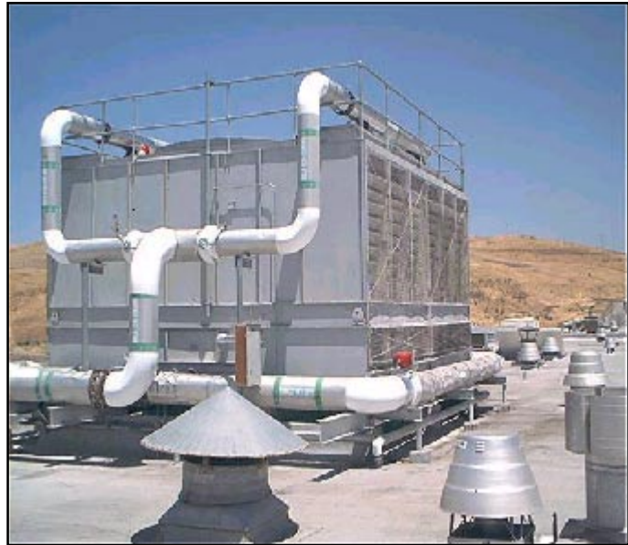
Modified central plant cooling tower installation features an 850-ton high efficiency chiller
