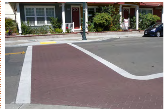
Pedestrian crossings can be highlighted with landscaped bulb-outs (top and middle) and special paving (bottom).
