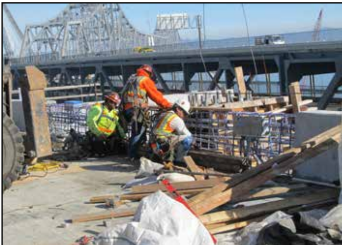
Yerba Buena Island Transition Structure Westbound Roadway Lighting Foundation Formwork and Conduit Installation
