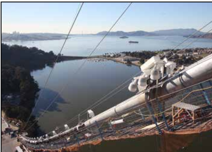
Self-Anchored Suspension Bridge Lighting Fixtures Installed on the Main Suspension Cable Back Span
