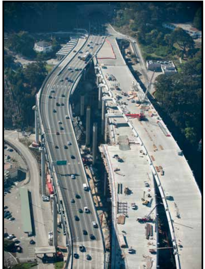
Ariel View of the San Francisco-Oakland Bay Bridge YBITS on the right and the Yerba Buena Island Detour on the left
