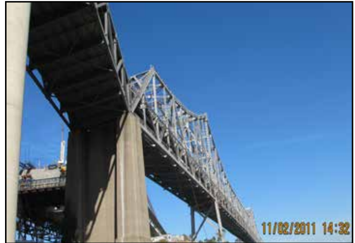
Dismantling Scope Included in the Future YBITS#2 Contract - YBI Detour E-1 column in center, Cantilever Bridge Deck at right
