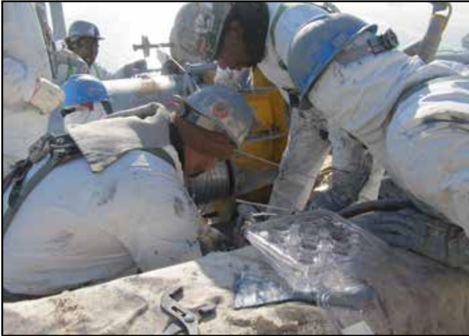
The San Francisco-Oakland Bay Bridge Self-Anchored Suspension Bridge Main Cable Wrapping Operations
