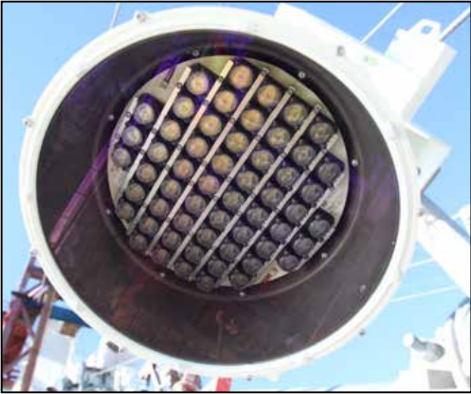
The Self-Anchored Suspension Bridge Newly Installed Light Fixtures
