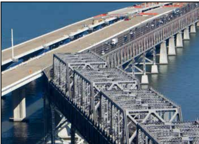
Existing San Francisco-Oakland Bay Bridge Segment to Be Dismantled in Future Contract(s)
