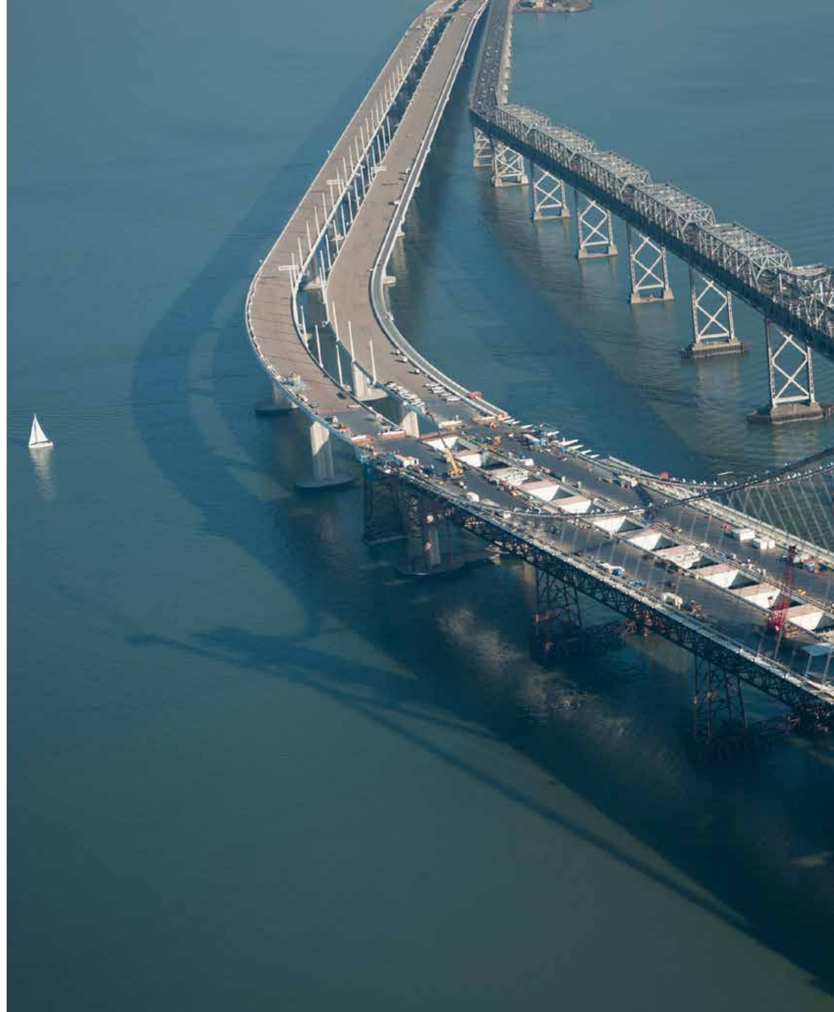
(Front Cover) The Self-Anchored Suspension Bridge Beginning the Placement of the Blue Main Cable Painting Enclosures
