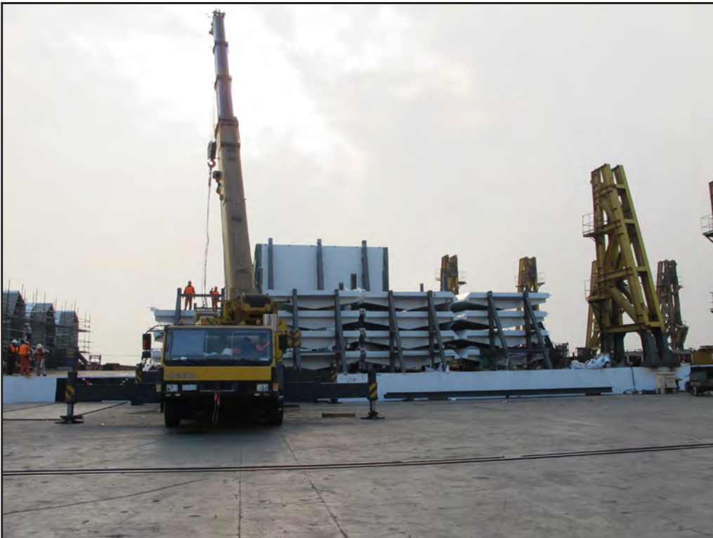
Bike Path Roadway and Cross Beam Being Prepared for Loading onto the Ship at ZPMC heavy Duty Dock in China
