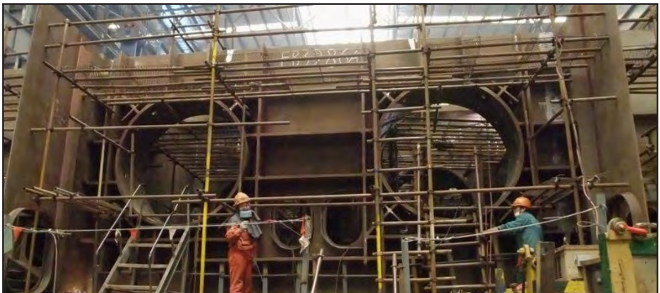
Hinge 'A' Floorbeams installed in Roadway Box 14 (East) at ZPMC in China
