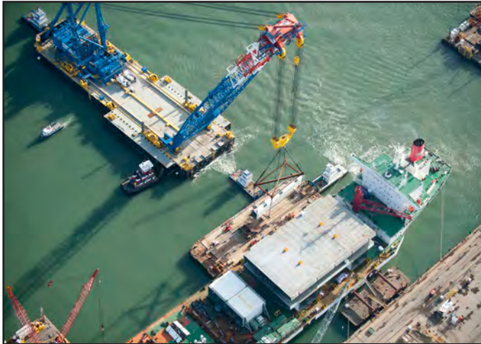
Shear-Leg Barge Crane Preparing to Offload Crossbeams and Roadway Boxes 10 East and West
