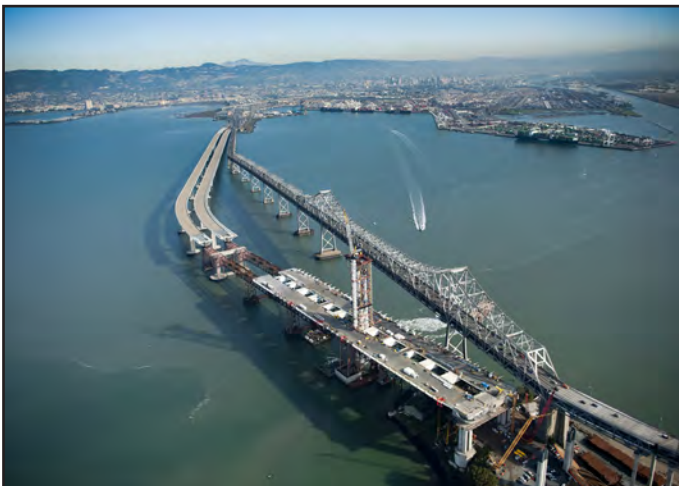
Aerial View of Tower Lift 3 Being Erected and Installed Roadway Boxes 1 through 9
