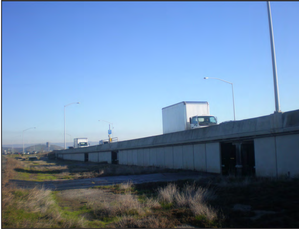
Curtain Walls Removed along West Approach for Preparation of Driving 48-Inch Diameter Piles
