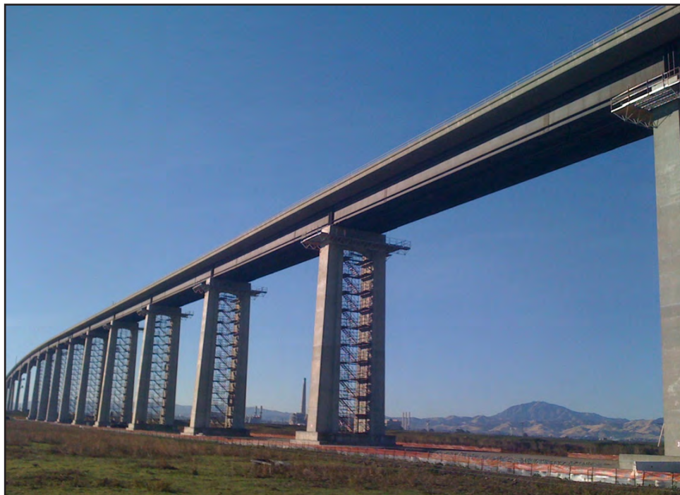
Piers Being Fitted for Construction Access Scaffolding to Allow for Drilling and Bonding of Reinforcing Steel at Cross-Frame Pedestals
