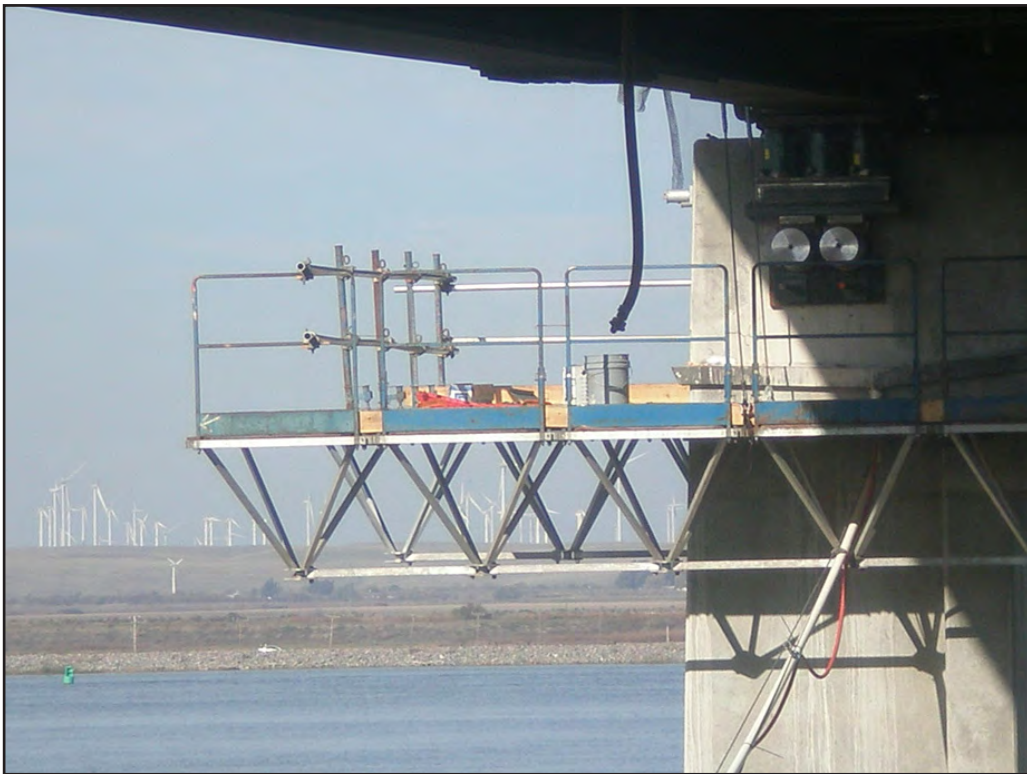
Work Platforms at Pier 7 and Jacks Installed under Girder Prior to Jacking
