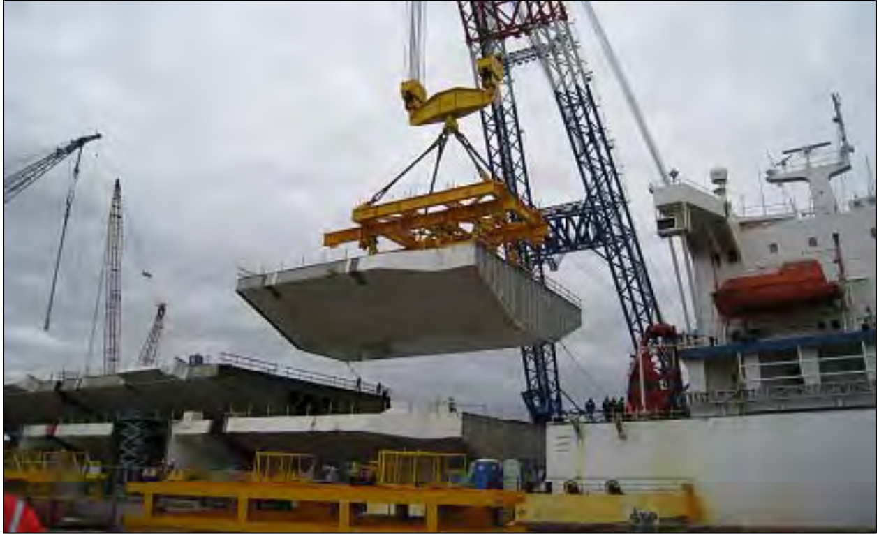
SAS Unloading of OBG Lift 1E
