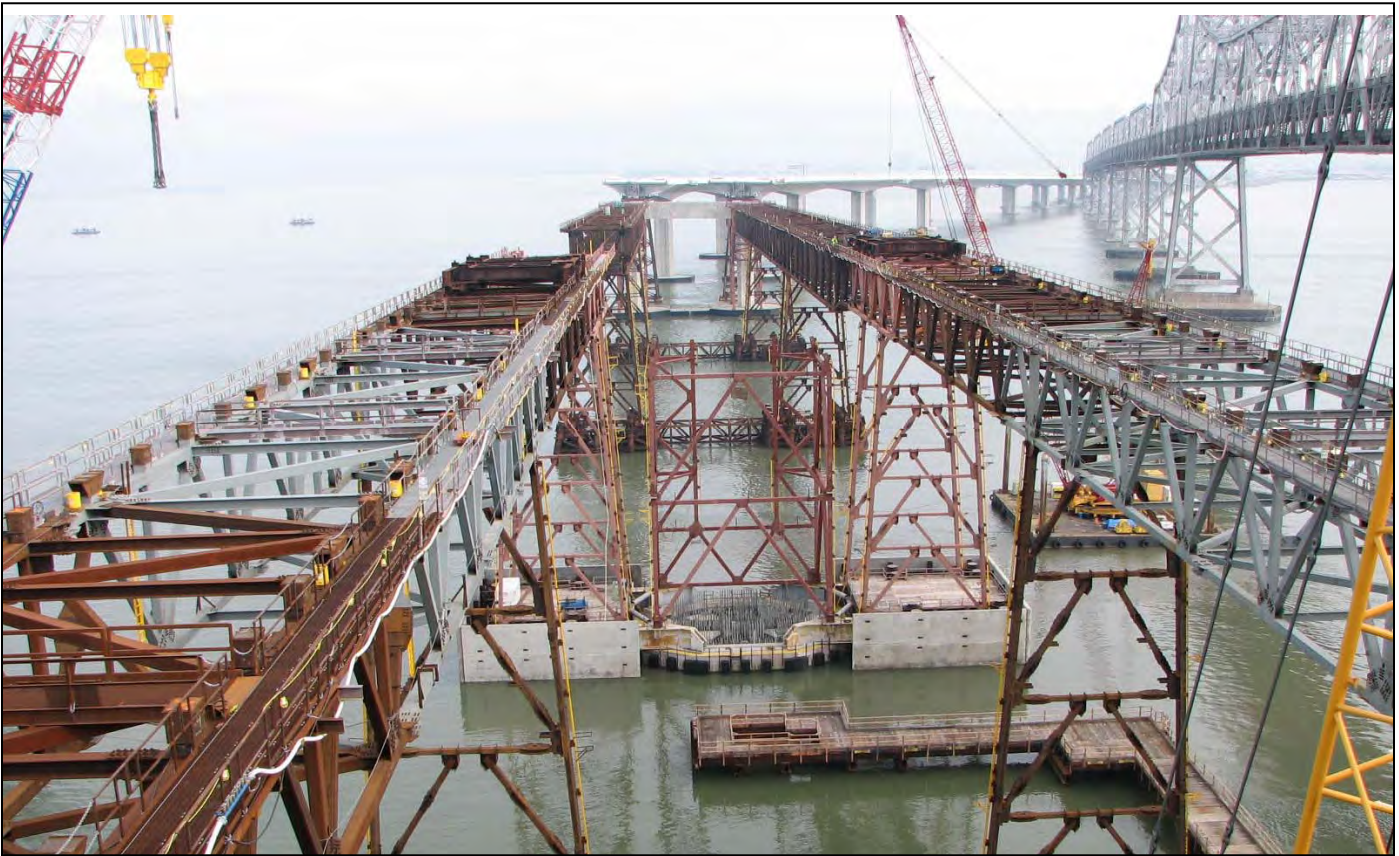
SAS Westbound and Eastbound Temporary Structures, T1 Erection Tower Framing and Trestle
