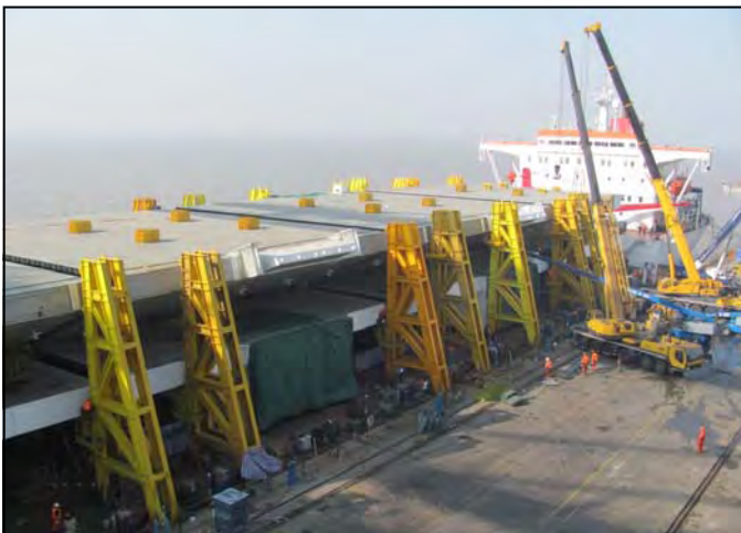
SAS Voyage 1 OBG Lifts 1- 4 East and West Loaded and Ready to Ship
