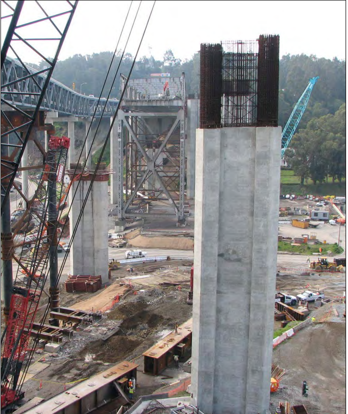
Yerba Buena Island Temporary Structures Column W3L and Demolition of Existing Viaduct Looking West
