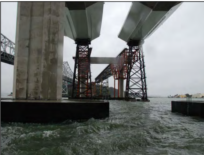
SAS - View from under the Completed Skyway Looking West towards Yerba Buena Island
