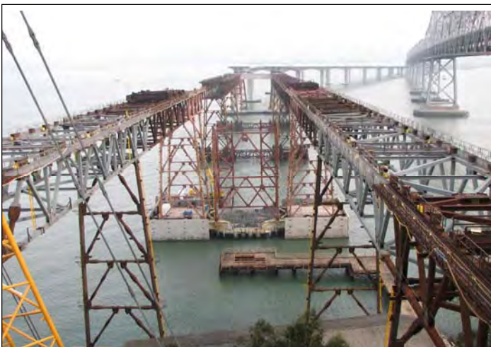
SAS OBG Cradles Erected on top of Westbound and Eastbound Temporary Structures
