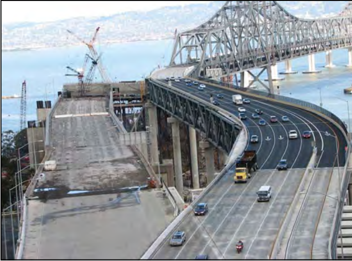
SFO Bay Bridge East Span Detour Structure Completed over the Labor Day Weekend
