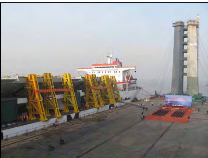
SAS Voyage 1 OBG Shipment and Tower Lift 1 Vertical Fit-up end of December 2009
