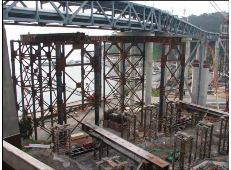
Yerba Buena Island Detour Skid Bent System and Beams Demolition in Progress
