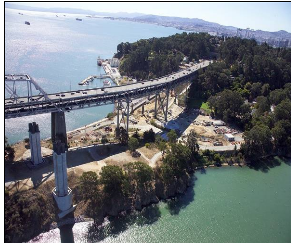
View of the completed W2 pier columns at the YBI, which will be the western support of the SAS structure
