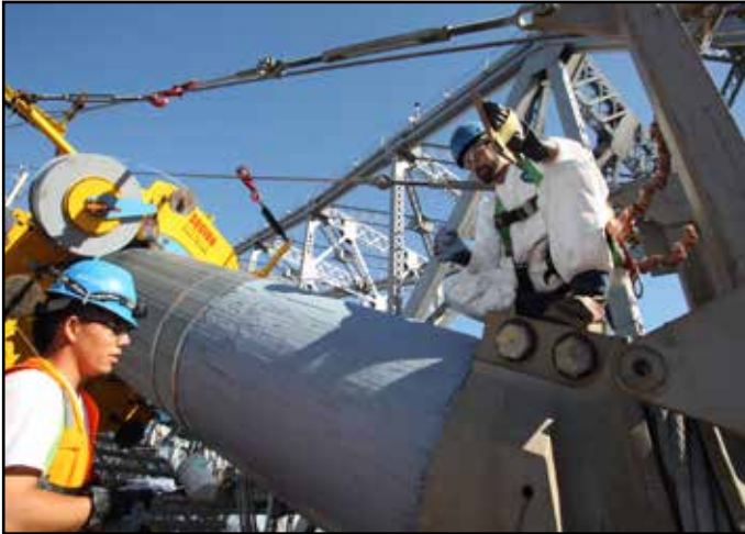
Self-Anchored Suspension Bridge South Back Span Zinc Paste Being Applied Prior to Cable Wrapping
