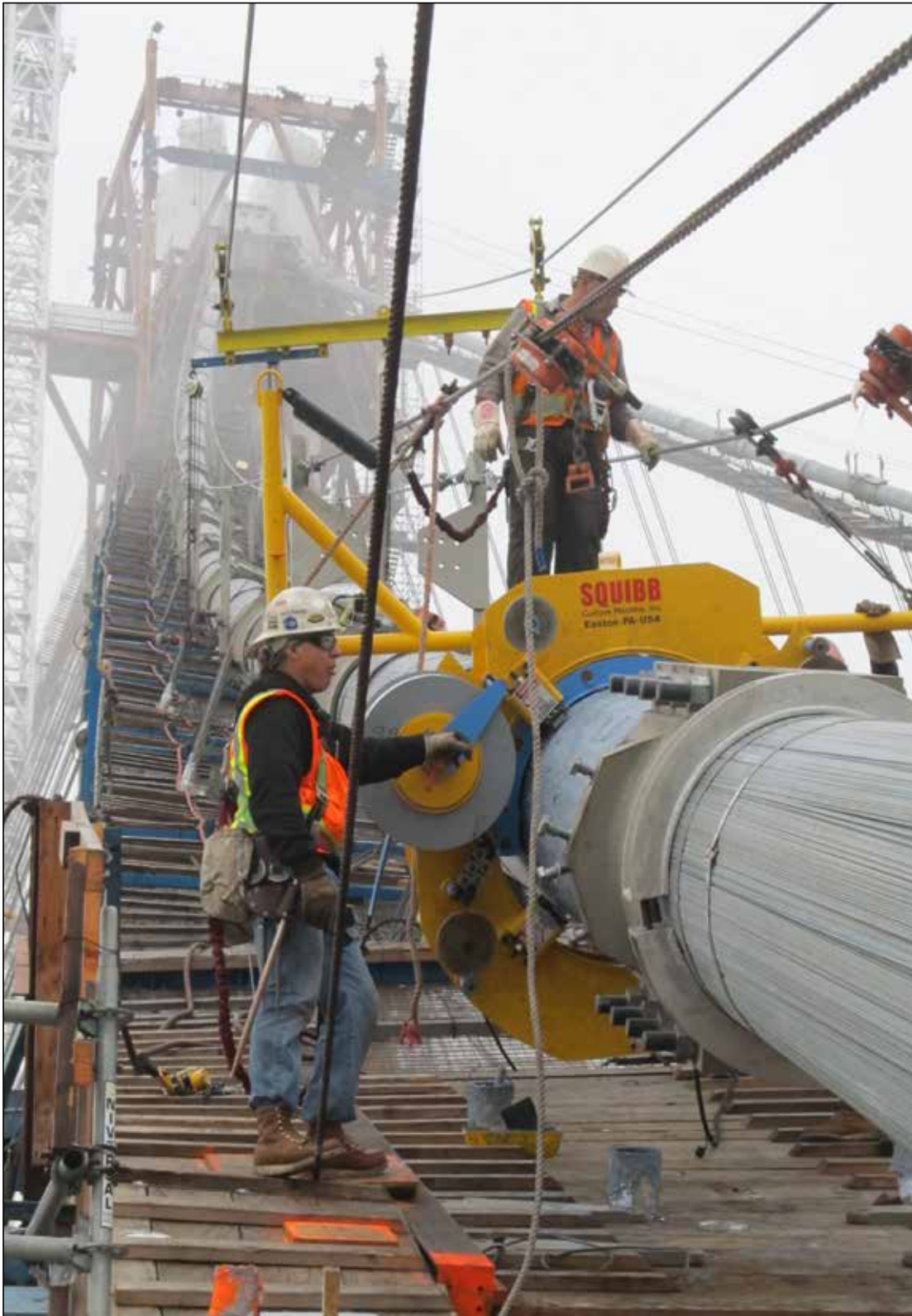
Self-Anchored Suspension Bridge Iron Workers Installing the Cable Wrapping Machine on the North Back Span Cable
