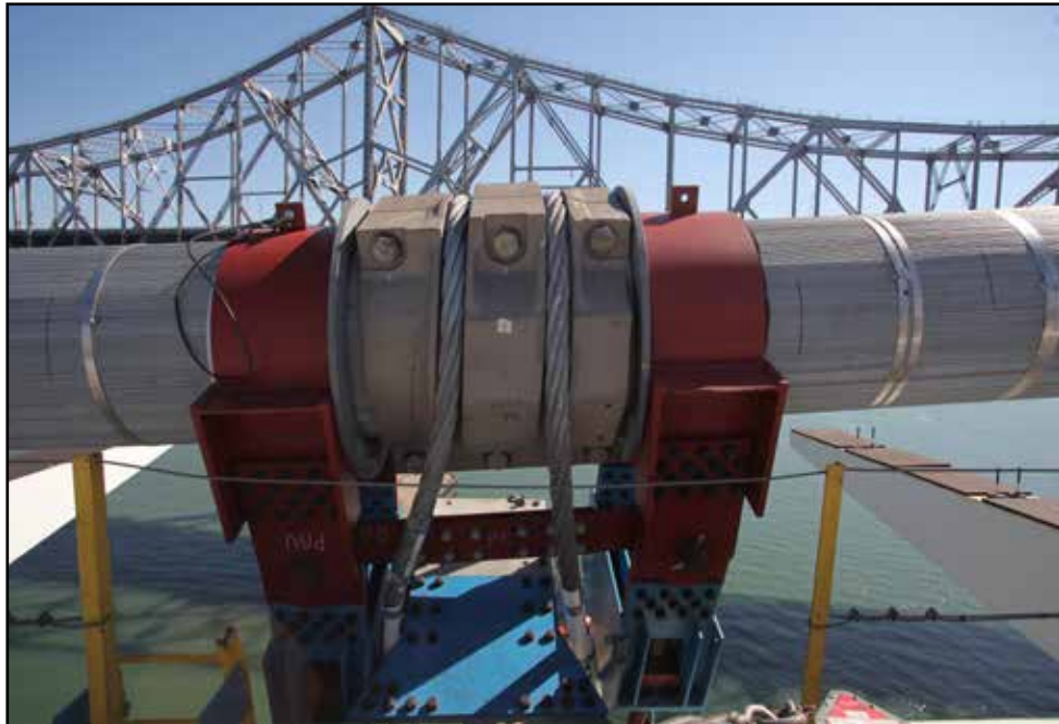
The Self-Anchored Suspension Bridge Cable Band and Suspenders Installed But Not Tensioned at Cable Swing-Out Location
