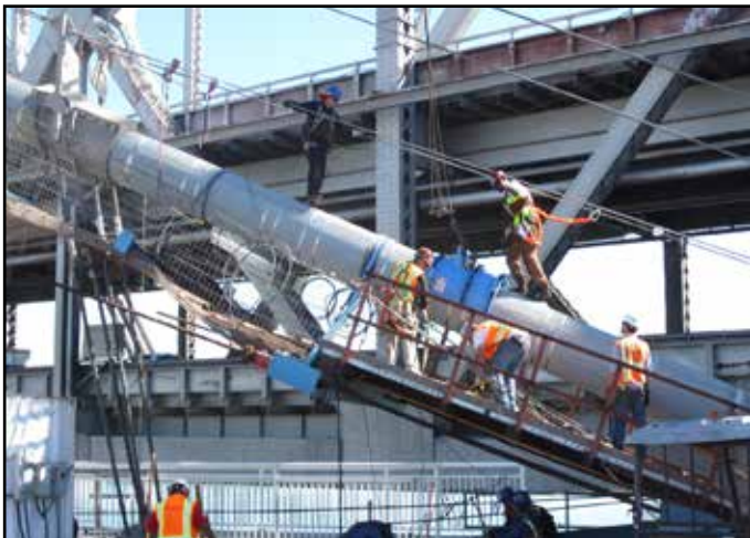
Self-Anchored Suspension Bridge Installing Cable Wrapping Skid Machine on South Back Span Cable
