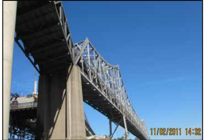
Dismantling Scope Included in the Future YBITS#2 Contract - YBI Detour at left, E-1 column in center, Cantilever Bridge Deck at right
