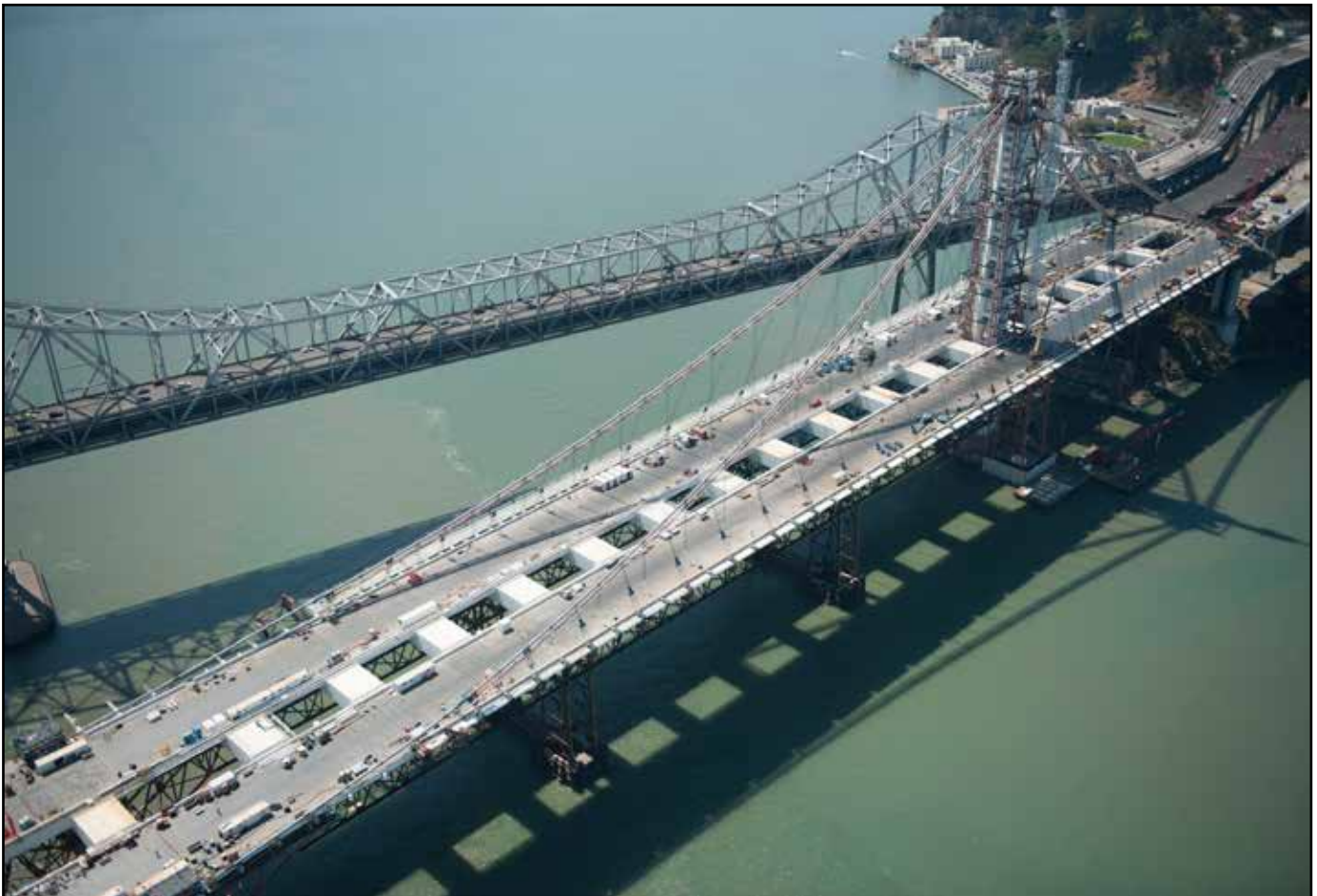
The Self-Anchored Suspension Bridge Tower and Roadway Deck Showing Suspender Cable Installation in Progress
