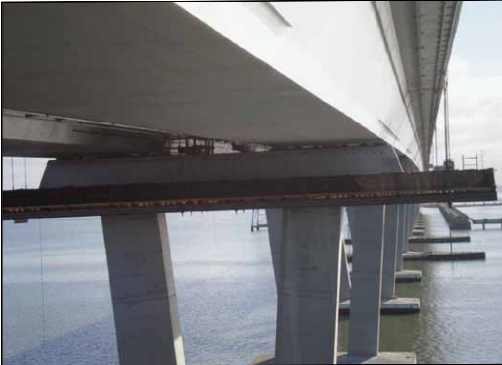
Dumbarton Bridge - Core Drilling of Bent Caps for Addition of Reinforcing Steel
