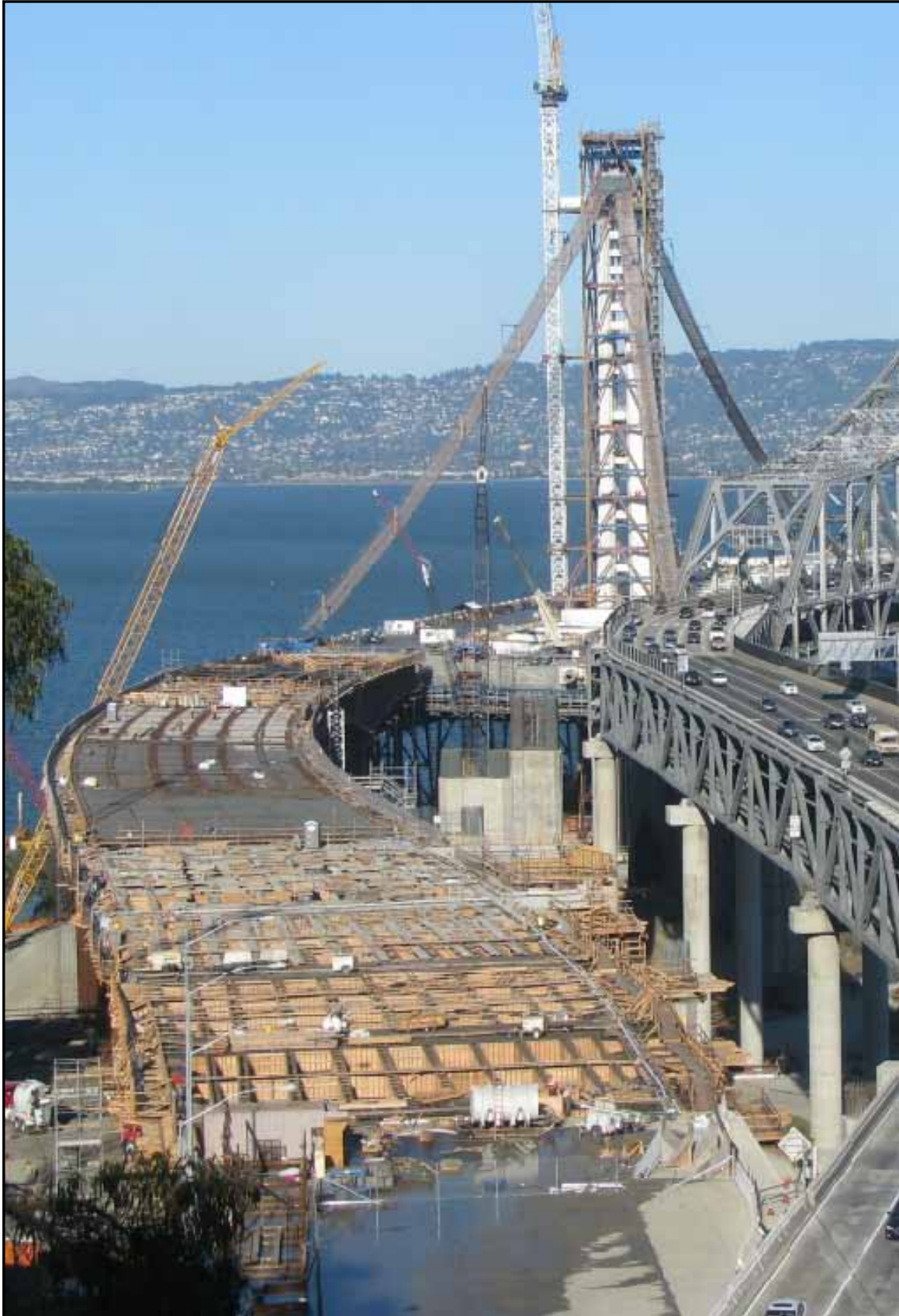
Overview of the Yerba Buena Island Westbound Transition Structure on left and Yerba Buena Island Temporary Detour on right
