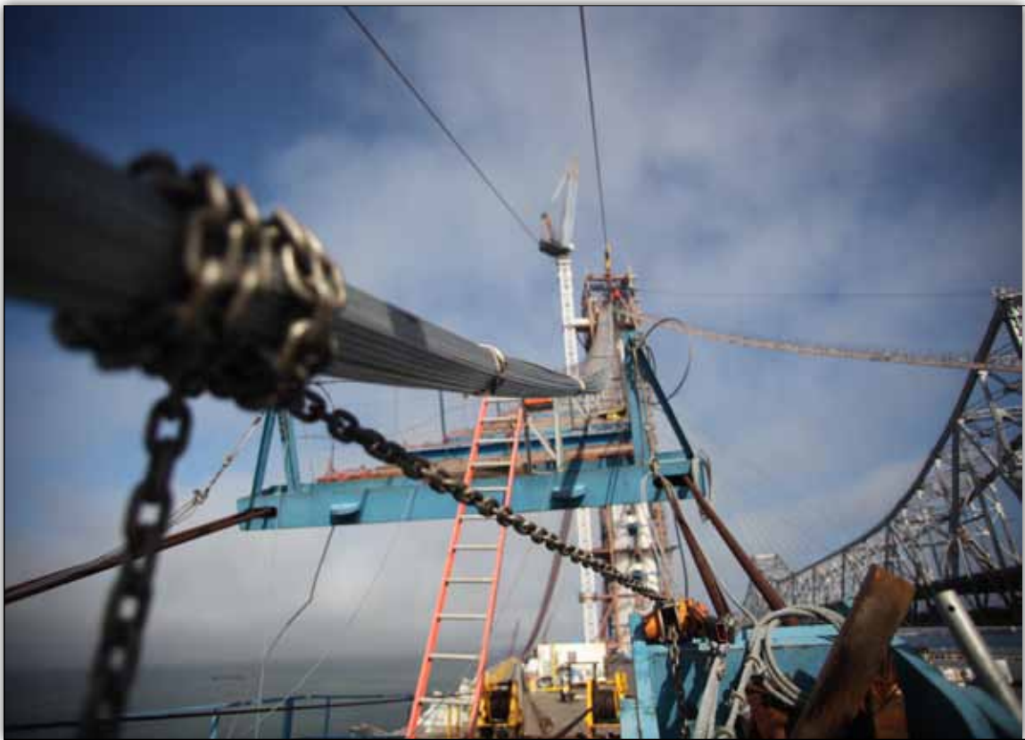
One Parallel Wire Cable Test Strand Being Hauled in Tramway System for Testing
