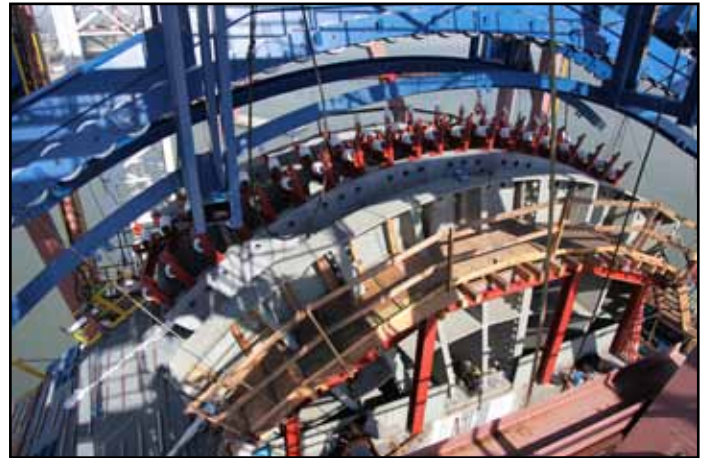
Self-Anchored Suspension Bridge Tower Saddle Area with Cable Tramway and Cable Installation Rollers in Place
