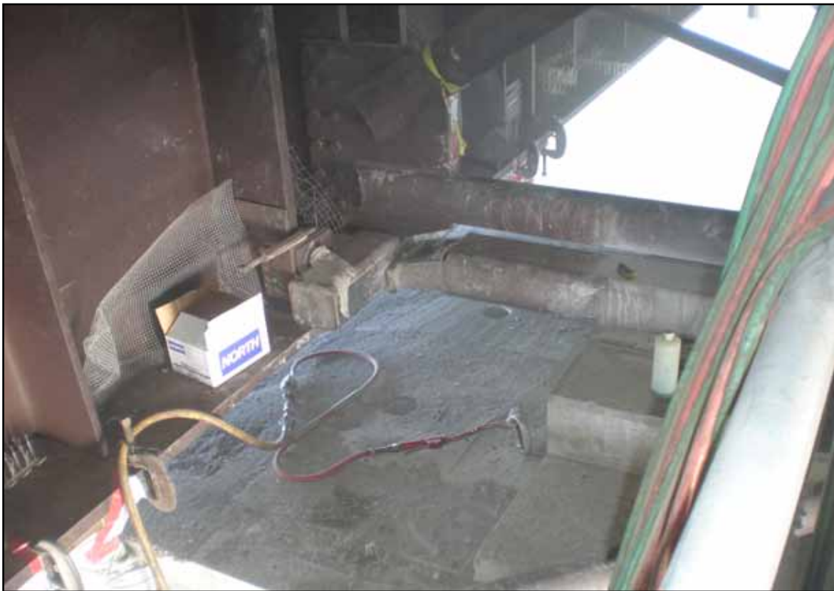
Pier 13 Concrete Removal is Necessary for Installation of the New Isolation Bearing
