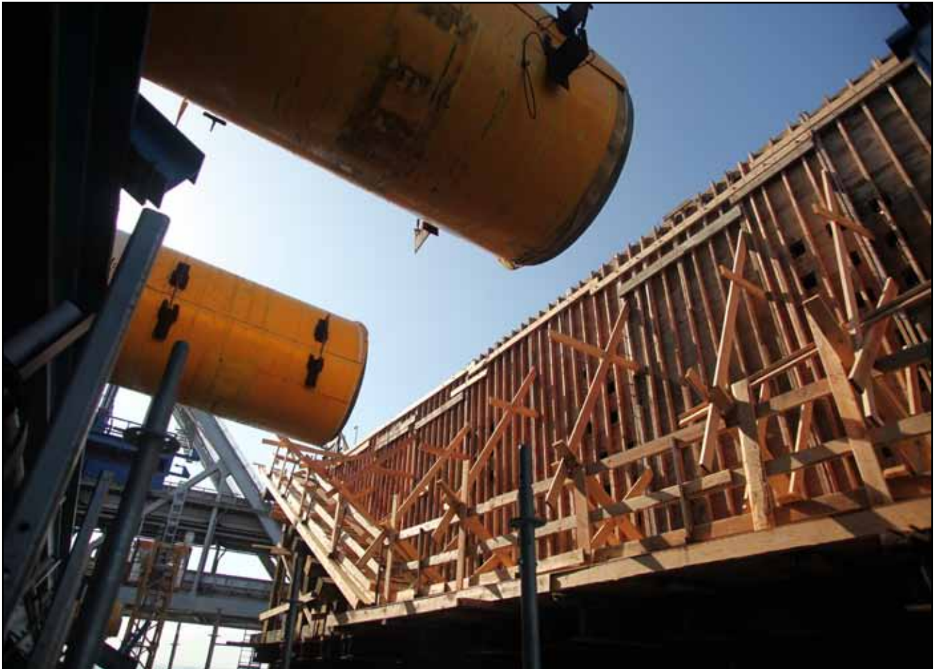
Hinge K Interface between the Self-Anchored Suspension Bridge and the Yerba Buena Island Transition Structure #1 Westbound
