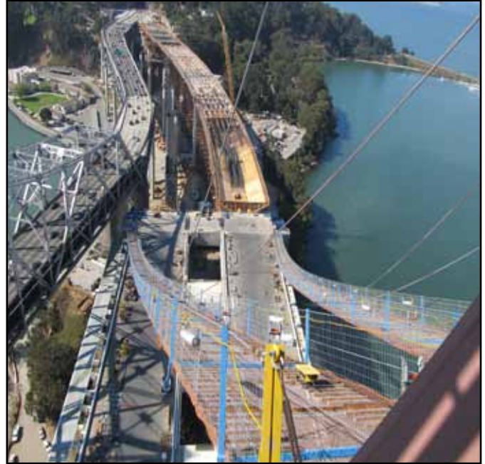
Overview of the Yerba Buena Island Westbound Transition Structure on right and Yerba Buena Island Temporary Detour on left
