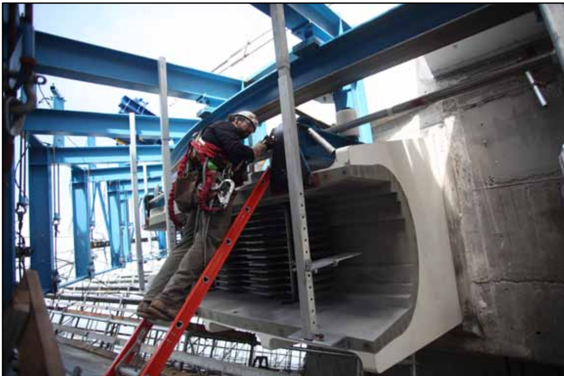
PWS Test Cable Strand Bundle Being Rolled above and around the West Deviation Saddle
