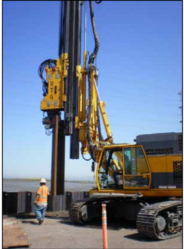
Steel Sheet Piles Driven for Cut-Off Walls for Installation of Drainage System and Flood Wall
