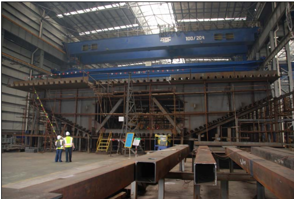
SAS – Box Girder Cross Section at the Zhenhua Port Machinery Company in China
