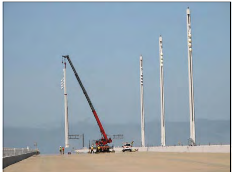
Sample Light Poles
