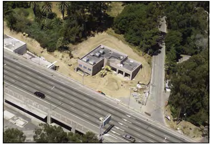
New YBI Electrical Substation
