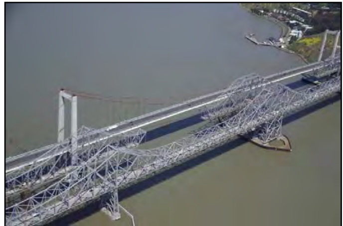
1958 Carquinez Bridge (foreground) with the 1927 Span (middle) under Demolition and the New Alfred Zampa Memorial Bridge (background)
