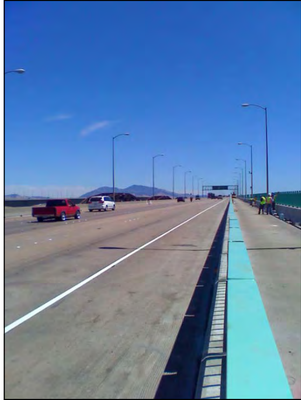
Completed Benicia-Martinez Installation of the Outside Rail Fence of the Bridge's Pedestrians and Bicycle Path
