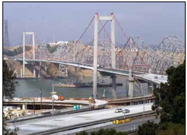
New Alfred Zampa Memorial (Carquinez) Bridge Soon after Opening to Traffic, with Crockett Interchange Still under Construction
