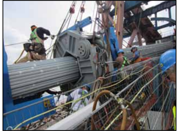
Maneuvering the Cable Compactor up to the Top of the Tower for Installation
