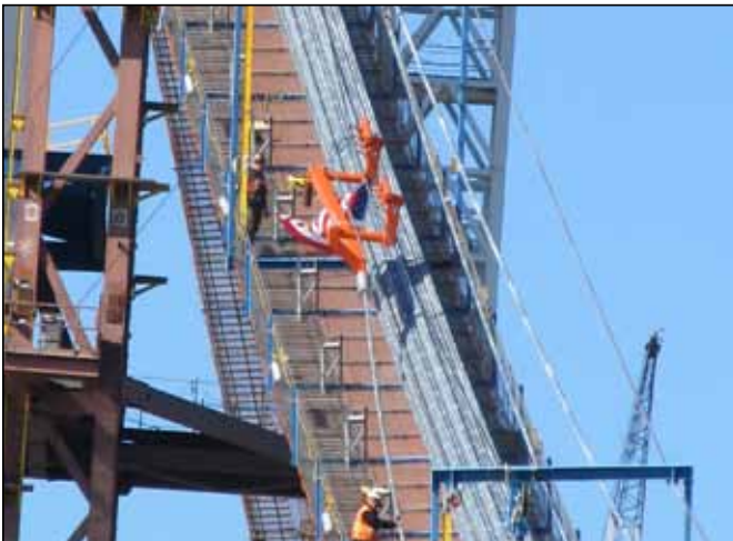
(3) Hauling Arm Pulling the PWS Cable Strand up to the Tower Saddle
