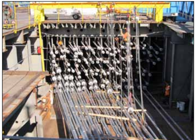
(4) Strand Haul Complete at Eastbound Anchorage Area and Connected to the Anchor Rods
