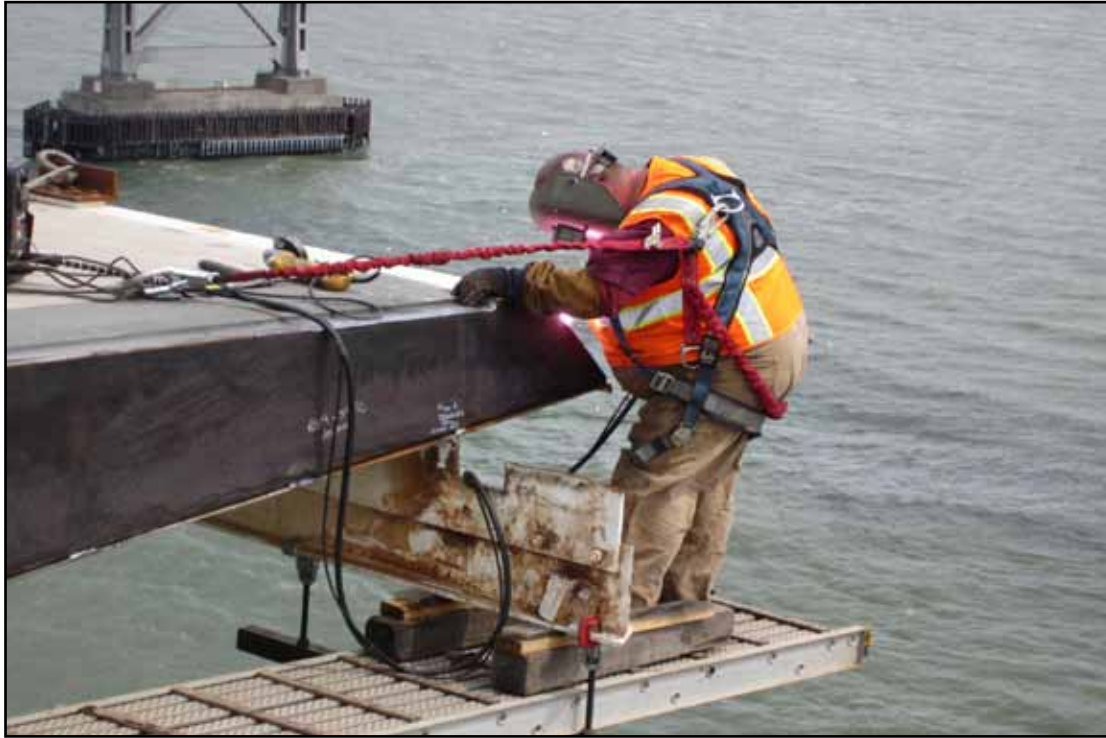
Welding Endplate at the Terminus of the Skyway Bike path at Trimming at Hinge A
