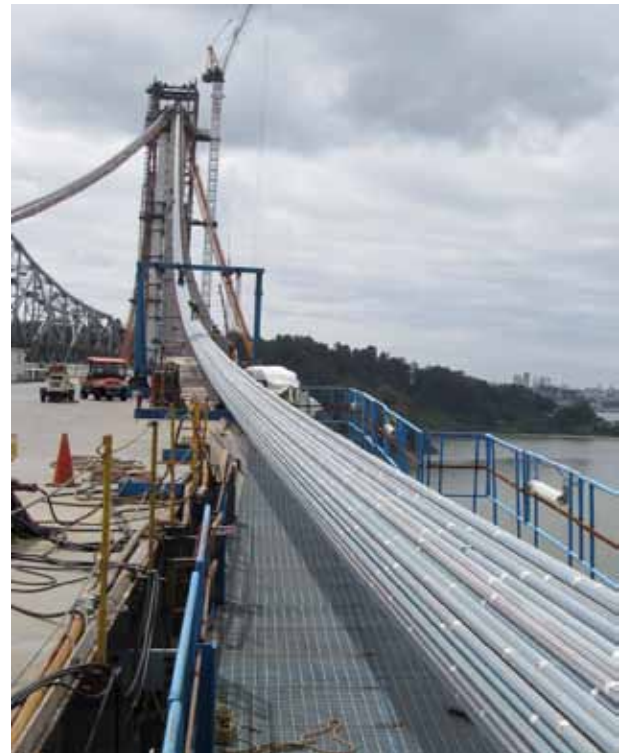
YBITS #1 Westbound Sections of Roadway on right with Existing Bridge and Yerba Buena Island Detour on Left with Hinge K at bottom right
