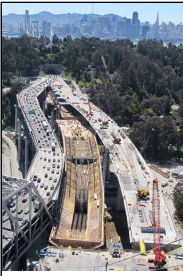
Yerba Buena Island Transition Structure #1 Westbound Deck Complete and Eastbound in Progress with Existing Bridge on Left
