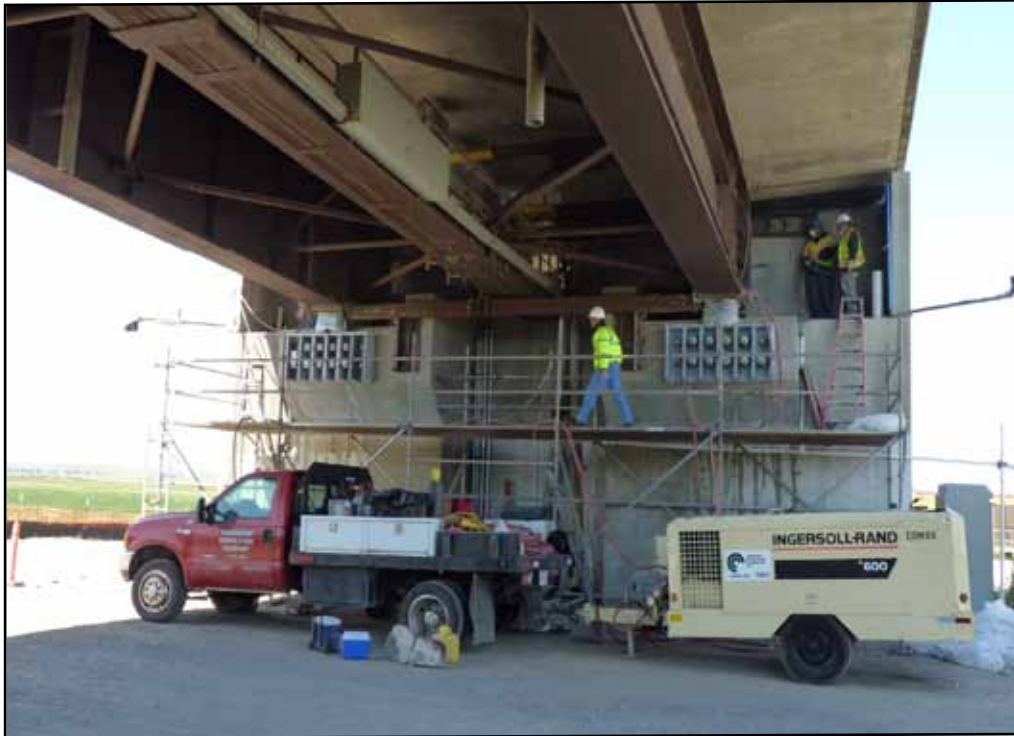
Antioch Bridge - Pier 41 Girders on Temporary Jacks prior to Installation of Isolation Bearings
