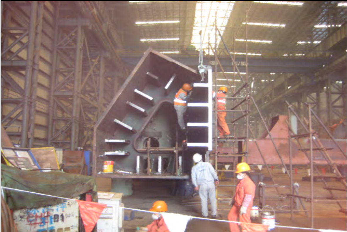
SAS - Internal Splice Plate Being Fitted to Skin D of Tower Box 4 East Shaft
