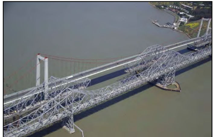
1958 Carquinez Bridge (foreground) with the 1927 Span (middle) under Demolition and the New Alfred Zampa Memorial Bridge (background)
