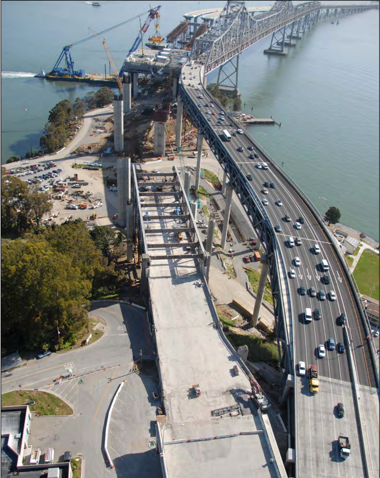
Existing Bridge Demolition Progress on Left, Temporary Detour on Right and Left Coast Lifter Placing a Roadway Box onto the Temporary Structures
