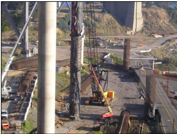
SoSoDet - Construction of columns for the viaduct portion of the Temporary Bypass Structure (TBS) adjacent to the U.S. Coast Guard Road on Yerba Buena Island
