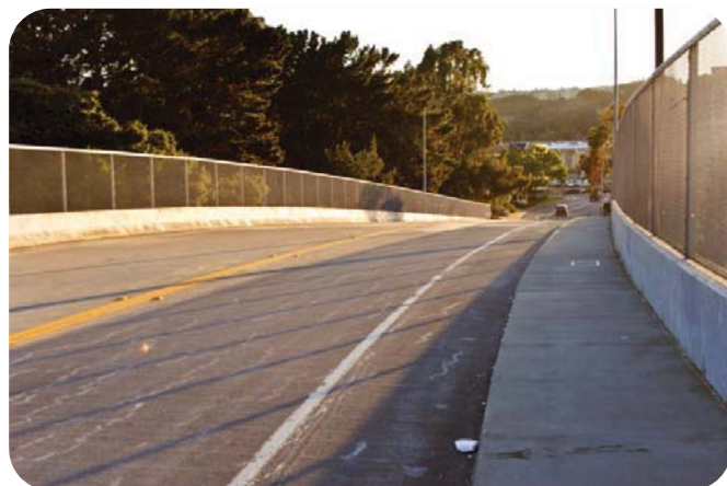
Sidewalks and bicycle lanes on the Merrydale Overcrossing are very narrow
