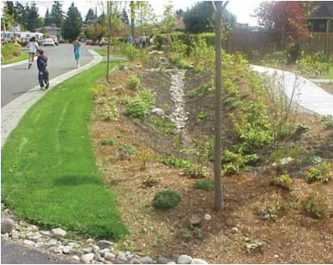
Swales can be used to add green space and treat flow control to reduce the burden on traditional utilities.
