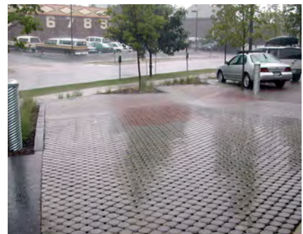
DG-41: Pervious paving allows infiltration of urban runoff and can provide an attractive design element.
