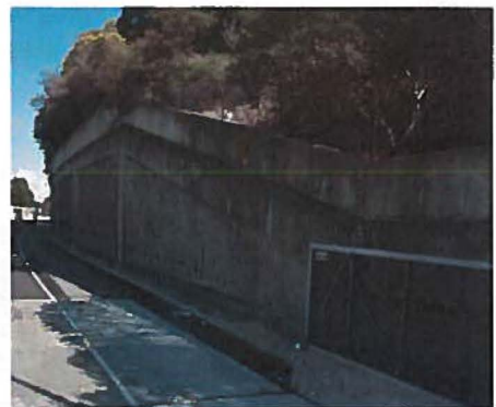
Eastbound I-580 requires widening in Contra Costa County to accommodate the third eastbound lane. The retaining wall shown must be removed and replaced with a wall set further back from I-580.
