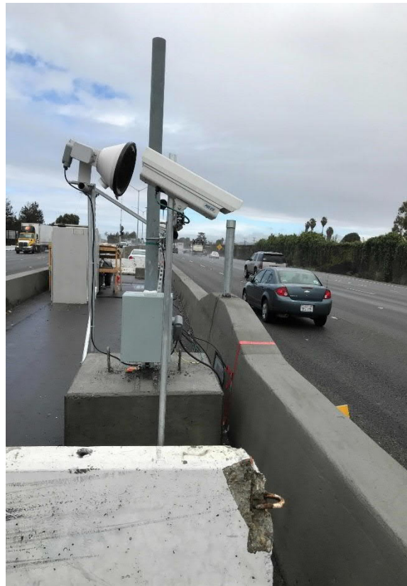
Figure 8: Example VOD equipment
