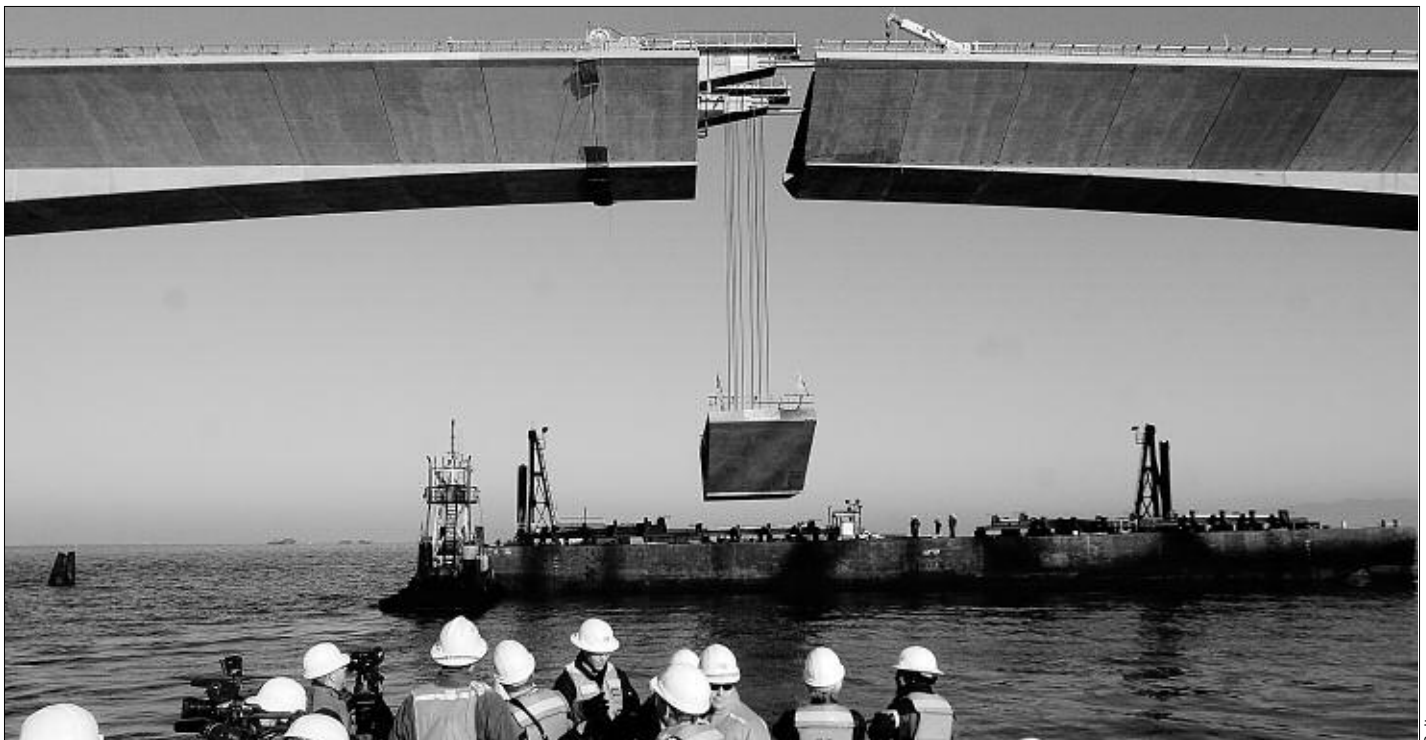
The last segment of the San Francisco-Oakland East Span Skyway is lifted into place.
