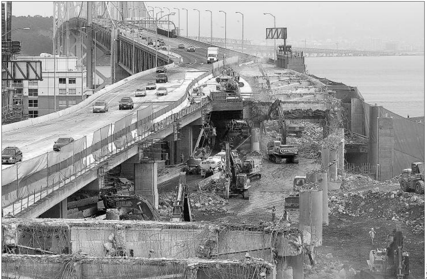
The old west approach to the San Francisco-Oakland Bay Bridge is demolished on Labor Day weekend, 2006.
