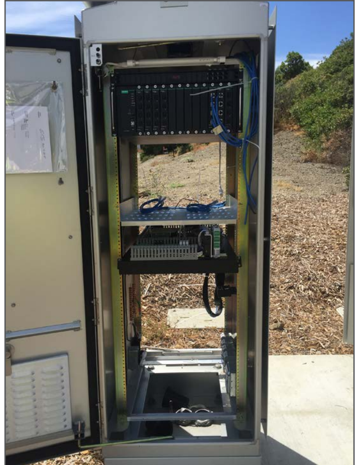
This roadside cabinet on I-680 houses the lane controller system, which provides monitoring, control, and management of each read point on a real-time basis.
