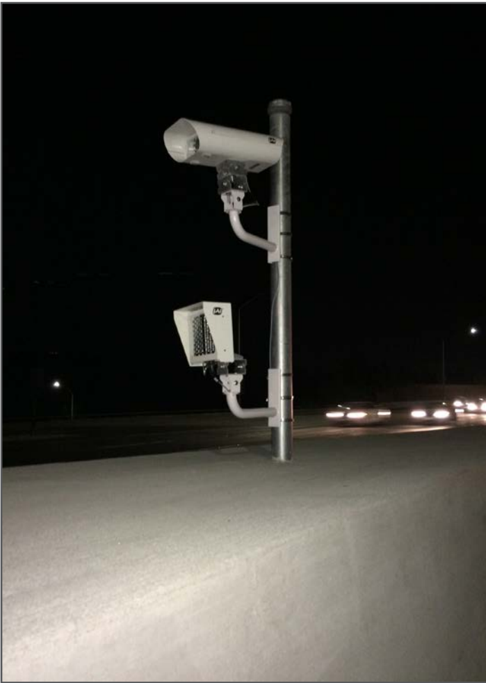
A Violation Enforcement System (VES) camera installed on I-680 to assist with express lanes enforcement.
