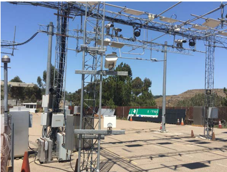
A test lane with all lane equipment at the toll system factory acceptance test.
