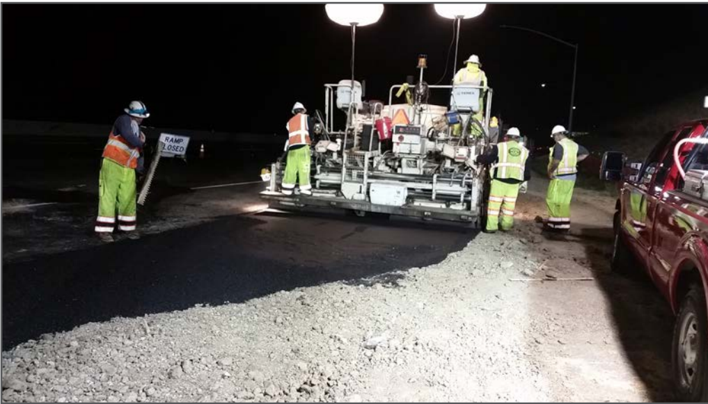
Construction crews paving an area for maintenance vehicles to service the toll equipment on I-680. The maintenance vehicle pull-outs will create a safer work environment for express lanes maintenance crews.
