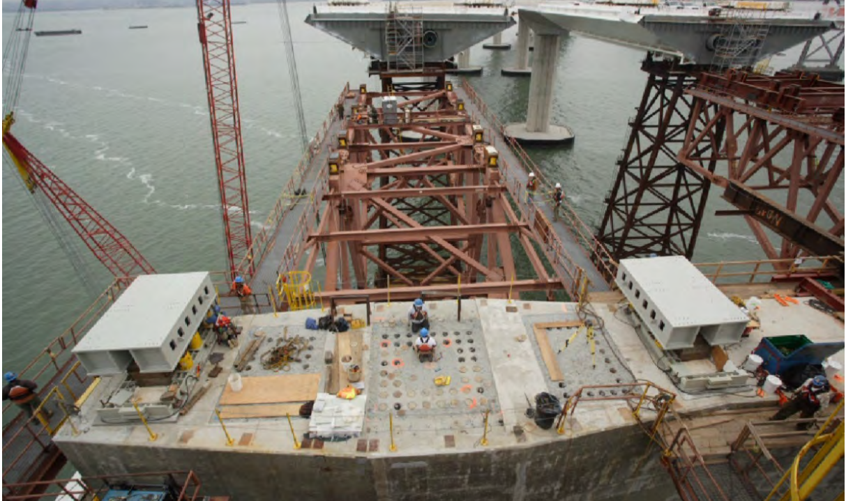
Figure 5 E2 Pier Cap Construction — (Center of photograph is the location of future shear key S1)
