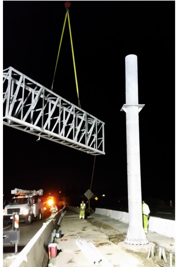
Construction crews secure a toll system sign post on I-680. Replacement of the median barrier will occur once the structural work is complete.
