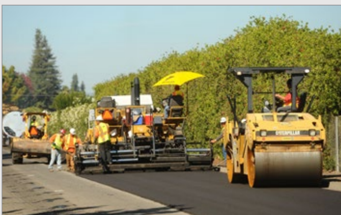
Two roadway sections resurfaced by recycling existing asphalt pavement in place, garnering a reduction in GHG emissions. (Photo: Noah Berger)
