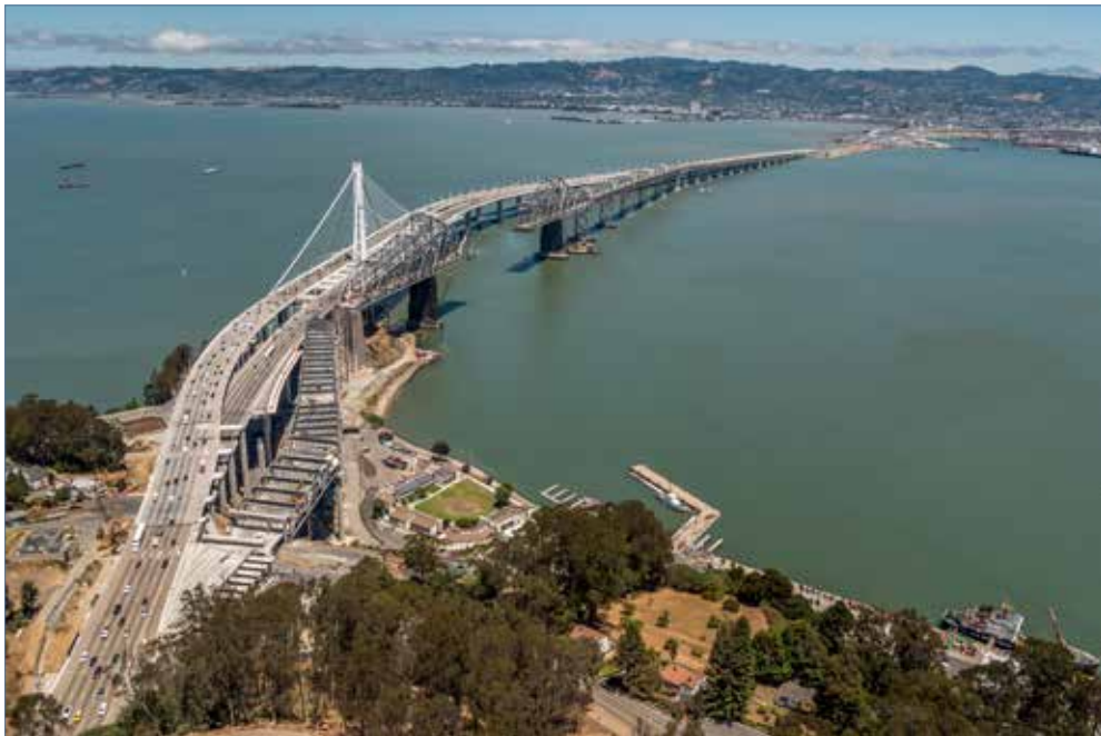
View Looking East to Oakland from the Tower of the Self-Anchored Suspension Bridge with Cantilever Demolition Progress on the right
