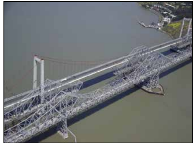
1958 Carquinez Bridge (foreground) with the 1927 Span (middle) under Demolition and the New Alfred Zampa Memorial Bridge (background)
