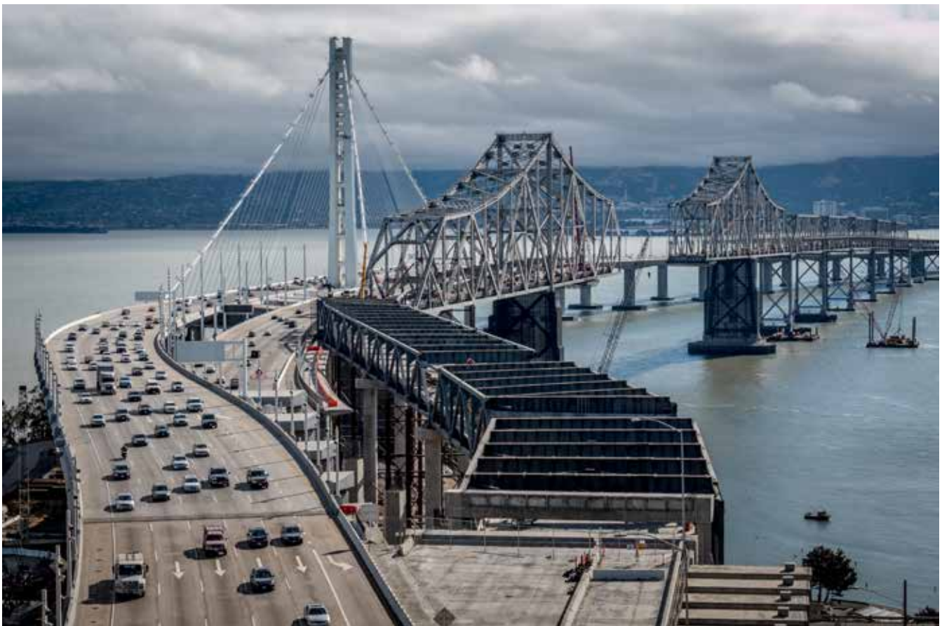
Eastern Span of the San Francisco-Oakland Bay Bridge on the left and Demolition Progress of the Old Bay Bridge on the right
